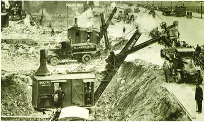
The basement of the present Conrad Hilton Hotel on Chicago's Michigan Avenue was excavated with these Bucyrus 20-B and 30-B steam shovels. Photo was taken about 1925.
